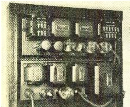
MOUNTED IN RACK Amplifier and power unit installed in rack frame
